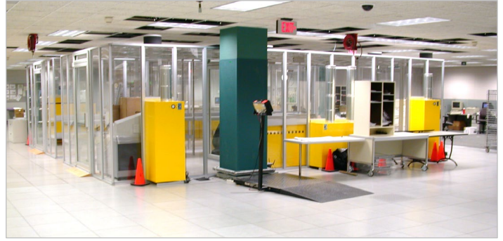
An example of a negative pressure room installation.
