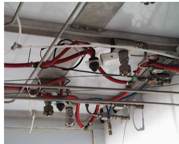
ESS nozzles in the chamber
